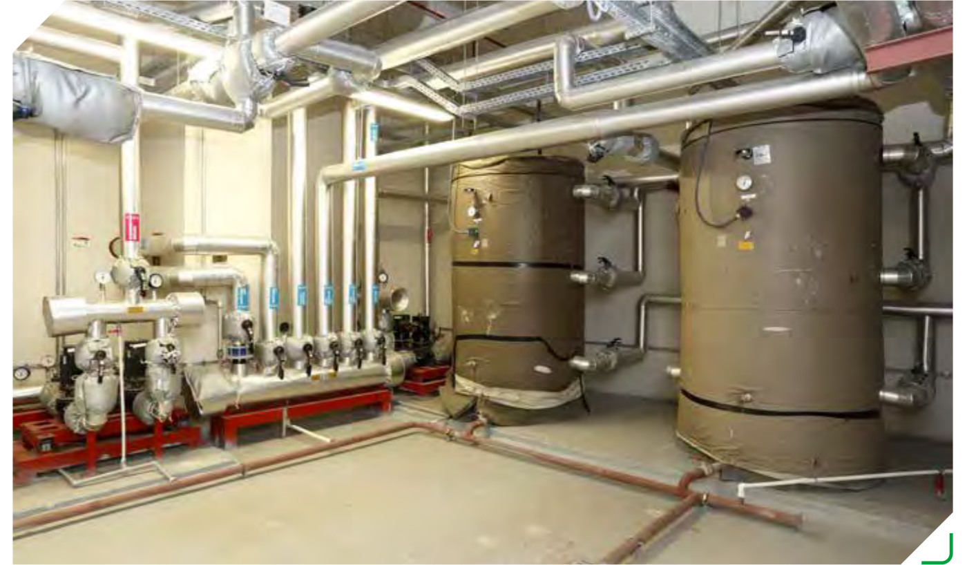
► Completion of mechanical and automation systems of a 5 stars hotel with construction area of 35.000 m 2 .
